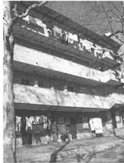
Photo 1. Trinitat Nova - a block of housing with severe structural weaknesses ( aluminosis ) (Photo: Montserrat Pareja Eastaway, 2003)
